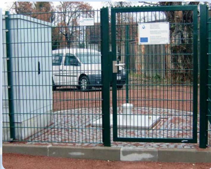
Pumpstation in Piethen
